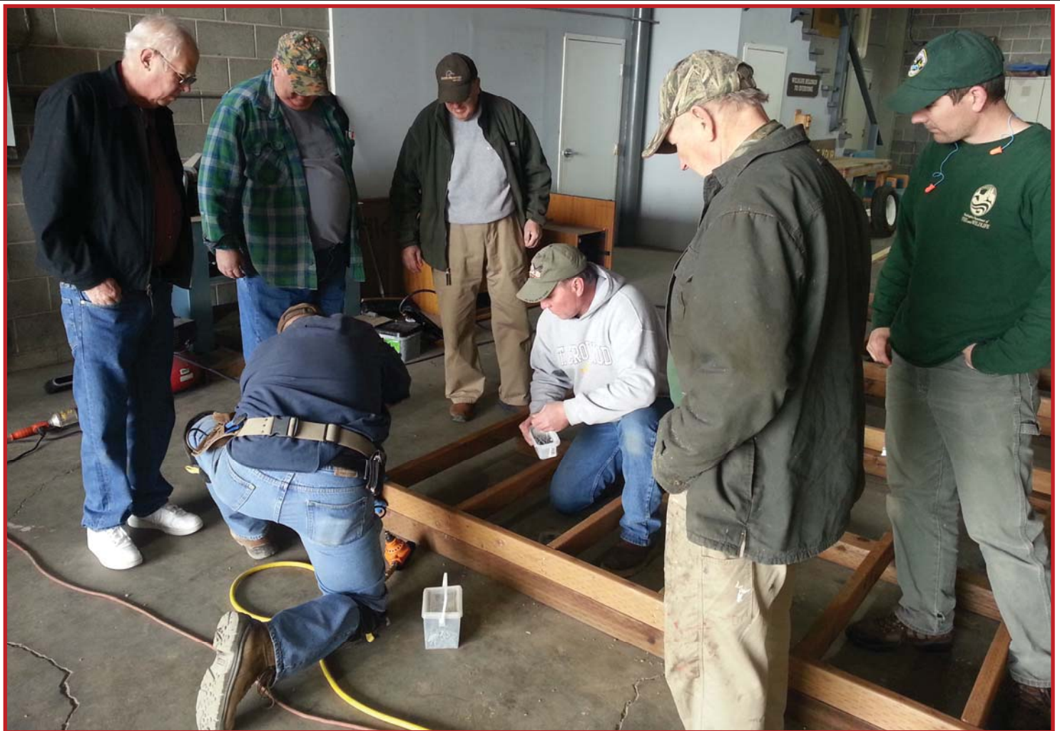
Too many cooks spoil the... At this stage of the process all one can really do is get out of the way of Bruce Feagan (ML) (on the floor, back to camera) using a special nail gun to secure metal braces in the corner sections of the floor foundation of this ADA capable hunting blind. From left include ML Chapter members, Robin Hickok, Dick Price, Col. Tom O'Dell, Jeff Waltz, Marvin Leyda, and WDFW's Asst. District Wildlife Biologist, Orrin Duvuvuei.
